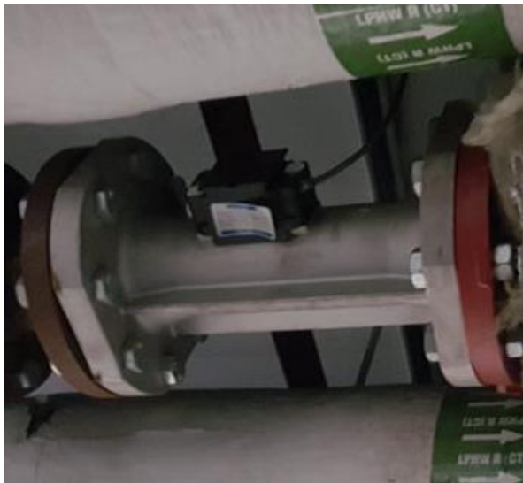
Ultrasonic flow measurement
