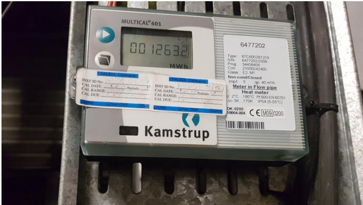
Kamstrup heat meter used in Charlestown
